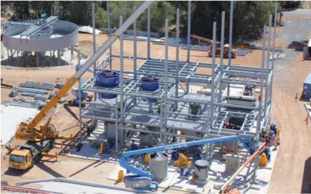
Work on the new chemical-grade plant as part of the Stage 2 Expansion at the Greenbushes Lithium Operations.
