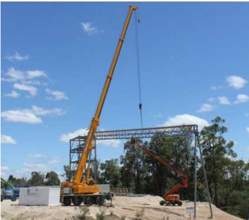
Conveyer belt to finished product stockpile being constructed as part of the Stage 2 Expansion at the Greenbushes Lithium Operations
